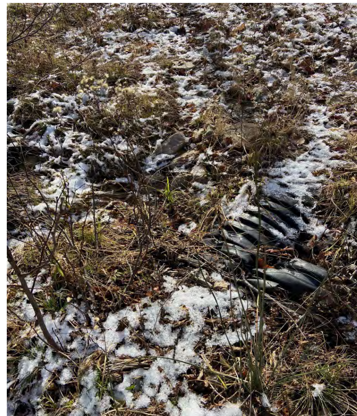
Photo 4: Feature 1 Crushed Culvert
