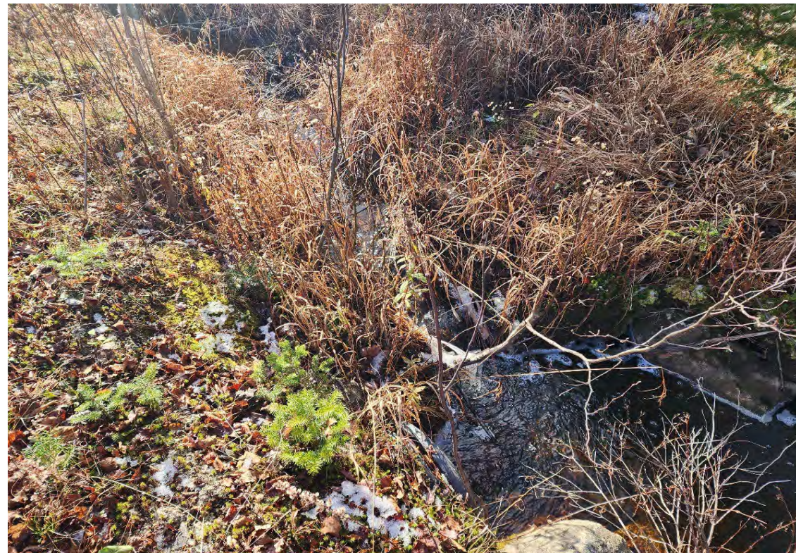
Photo 3: Sunken Culvert D/S of crossing
