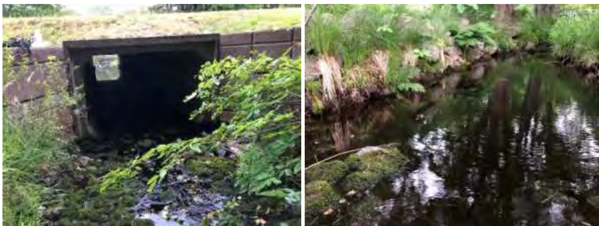
Figure 13. Unnamed tributary that becomes well defined before flowing through a concrete culvert under Upper Clyde Road and entering the Roseway River, July 8, 2020.
