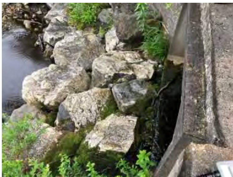
Figure 35. Outlet of culvert of unnamed tributary at Upper Clyde Road and Roseway River, July 8, 2020.
