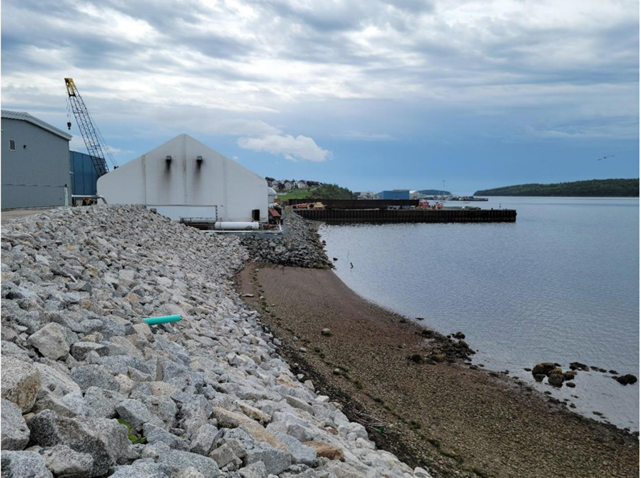
Proposed treated effluent discharge location, adjacent existing discharge point from on-site storm water separator (First Defence®) system (photo date: September 2021).
