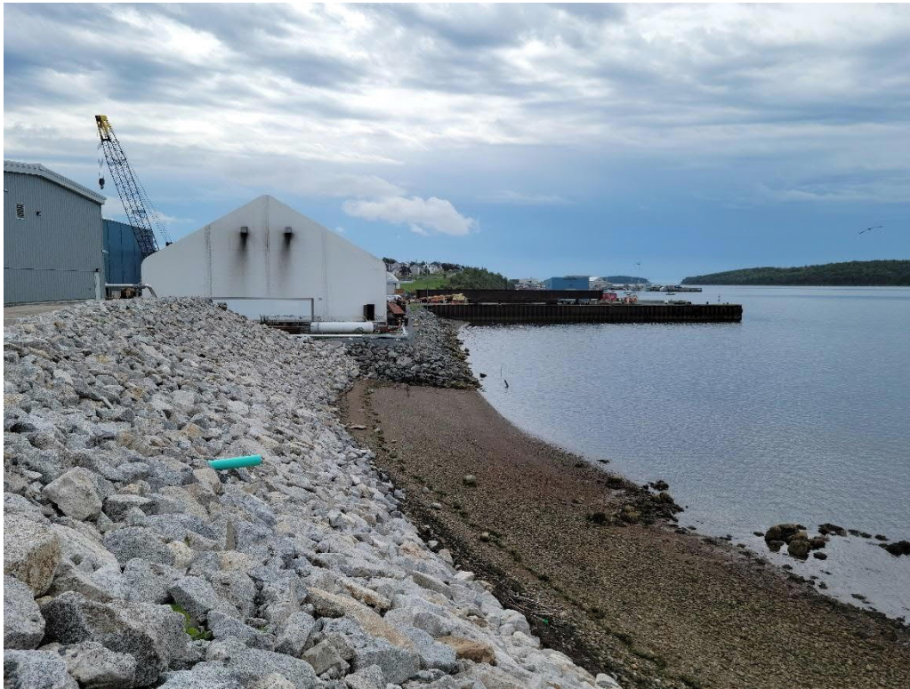
Figure 1: Armour stone installation at the project site, with discharge pipe (photo dated September 2021)
