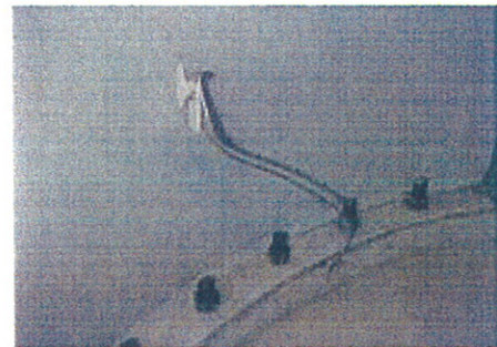
Fig. 5: Connection between steel tower and foundation earth electrode
