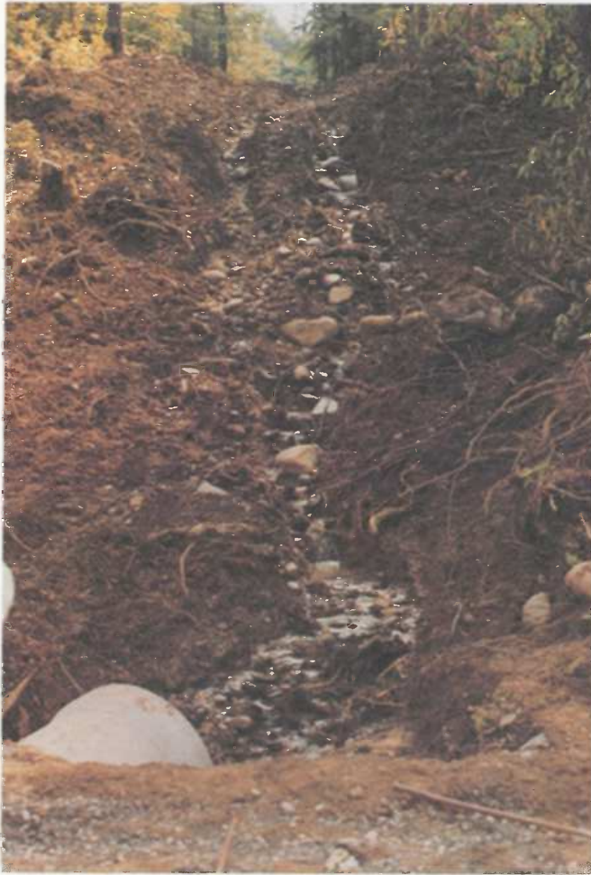
Good example of a riprap-lined chute. Before: an unstable and eroding slope.
