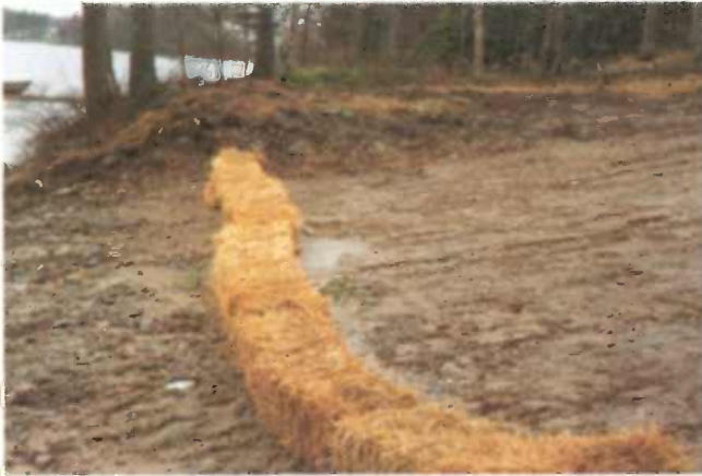
Straw bales used to filter sediment near the edge of a lake — here, one small lot is being developed.
