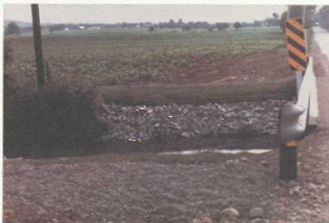
Riprap, sod and crushed stone used to stabilize stream bank after installation of a pipe line.
