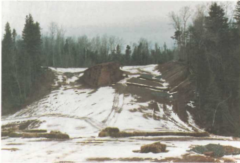
Roadway being built over a brook. Straw barrier intercepts sheet flow, diverting it to a temporary siltation
