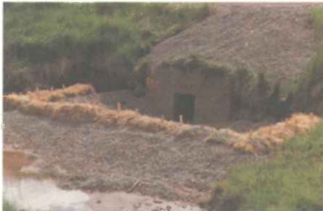
Here, the straw bales are covered with crushed stone and used as a berm to filter runoff from a large construction area before it flows off the site into a storm sewer.
