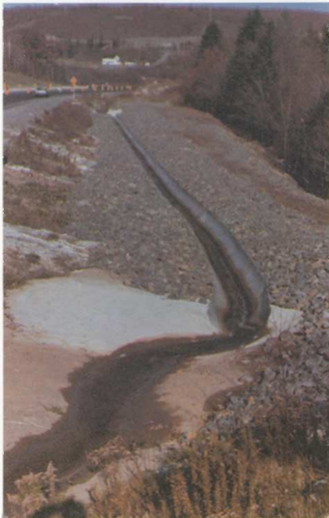
Good example of a corrugated steel pipe down drain.
