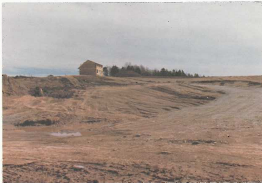
Figure 2: A housing development where vegetation has been completely stripped, exposing bare soil to rainfall erosion on a long, steep slope.
